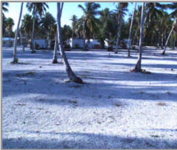
Lack of coral fill between newly constructed garages and original resettlement camp.
