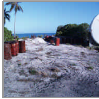
Mounds of soil and unscrapped surfaces around debris piles and construction materials, tanks.
